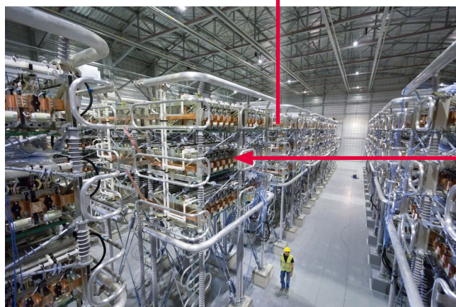
Source: Siemens AG Typical Voltage Source Converter Installation
